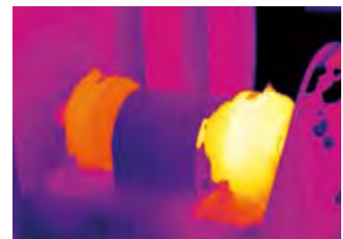
Overheating bearing cap
